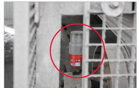
Lubrication of pillow block on a tail pulley
