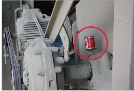
Lubrication of pillow block on a drive pulley
