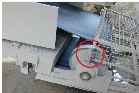
Lubrication of pillow block on a conveyor
