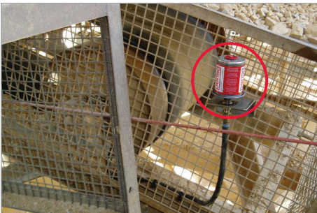
Lubrication of pillow block on a conveyor
