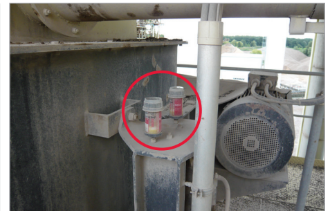
Lubrication of pillow block on a conveyor
